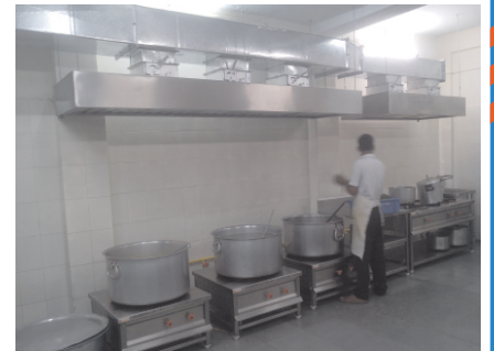
Kitchen Exhaust Hood & Ducting
