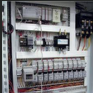
PLC AND SCADA , MCC PANEL
