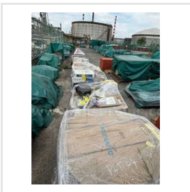
MRO From Petrochemical Refinery
