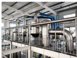
Three Phase Liquid Extraction Plant
