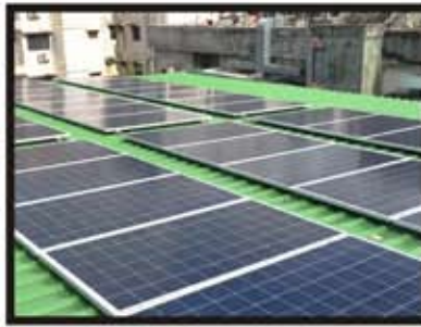
20 KW at Pulse Imaging & Diagnostic Centre, Nagpur
