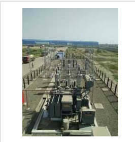
Electrical Transformer Installation Services
