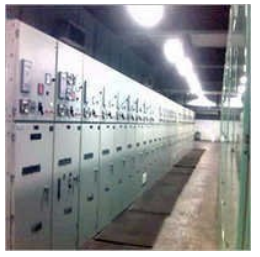
Panel Installation Services
