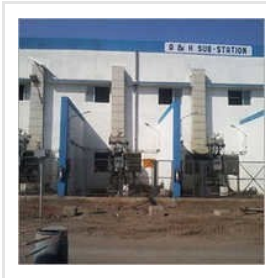
Power Transformer Installation Services
