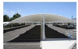
Car Parking Shade Structure
