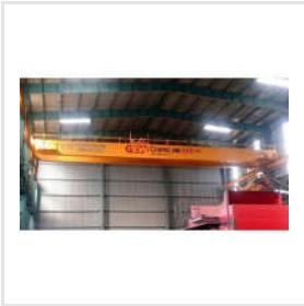
Double Beam EOT Crane
