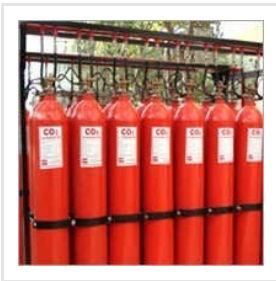
Gas Flooding System
