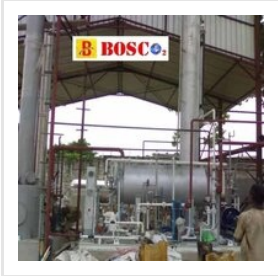
CO2 Generation Plant
