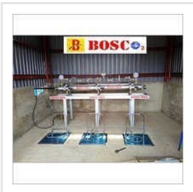
CO2 Filling Station
