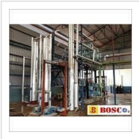
CO2 Gas Recovery Plant
