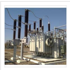
Substation Transformer Service
