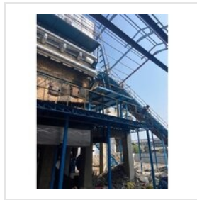
Plastic Fired Boiler
