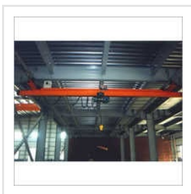
Under Slung Crane
