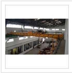
Double Girder Overhead Crane
