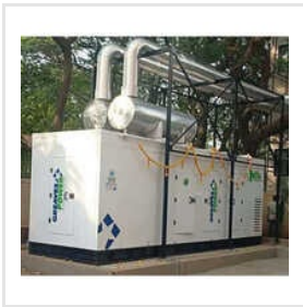
1010 Kva Diesel Generators
