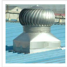
Rooftop Air Ventilator
