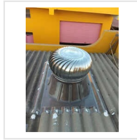
Rooftop Air Ventilator
