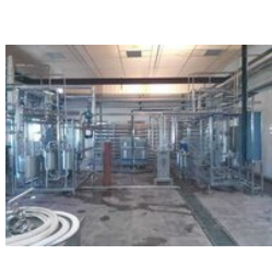
Milk Processing Plant
