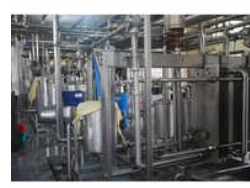
Milk Processing Plant And Machines
