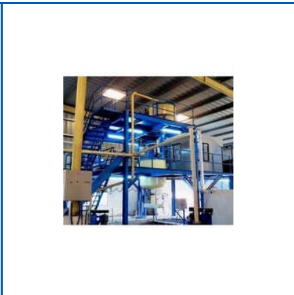
AAC BATCHING PLANT
