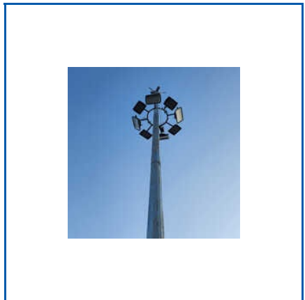
LED FLOOD LIGHT HIGH MAST POLE
