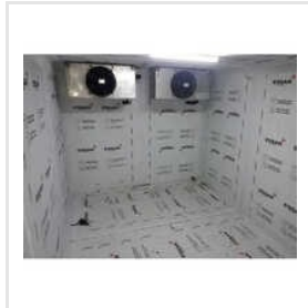
Medicine Cold Storage Room
