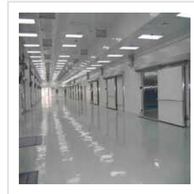
Commercial Cold Storage Room
