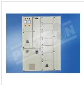
Main Power Distribution Board
