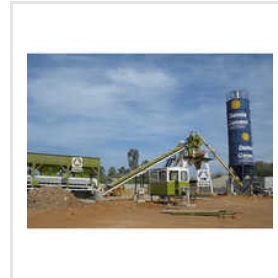
Industrial Stationary Concrete Batching
