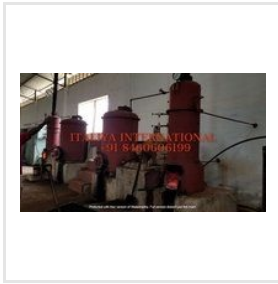
RCN Cooking Cashew Steam Boiler
