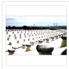
Industrial Wind Ventilators
