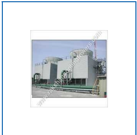
EVAPORATIVE COOLING TOWER
