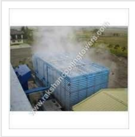
Natural Draft Cooling Towers
