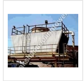
Industrial Wooden Cooling Tower
