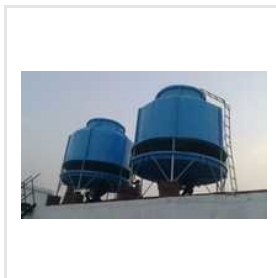
200 TR Cooling Towers
