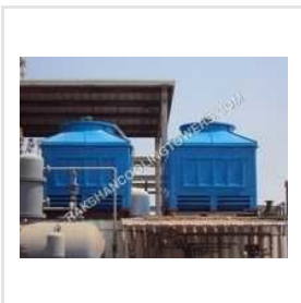
Square Cooling Towers
