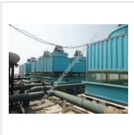
Cooling Towers Suppliers In Guntur
