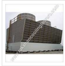
Timber Cooling Tower
