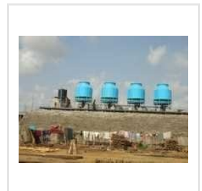
100 TR Cooling Towers
