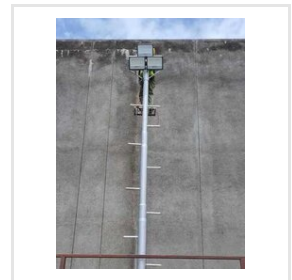
Solar Street Light Pole
