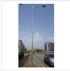
High Mast Lighting Pole
