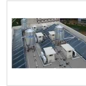
Industrial Heating System
