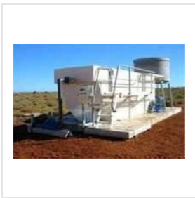
Sewage Water Treatment Plant
