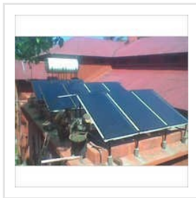
Solar Hot Water System
