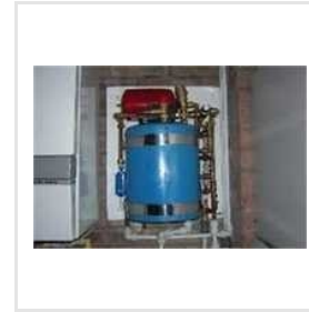
Boiler Air Preheater
