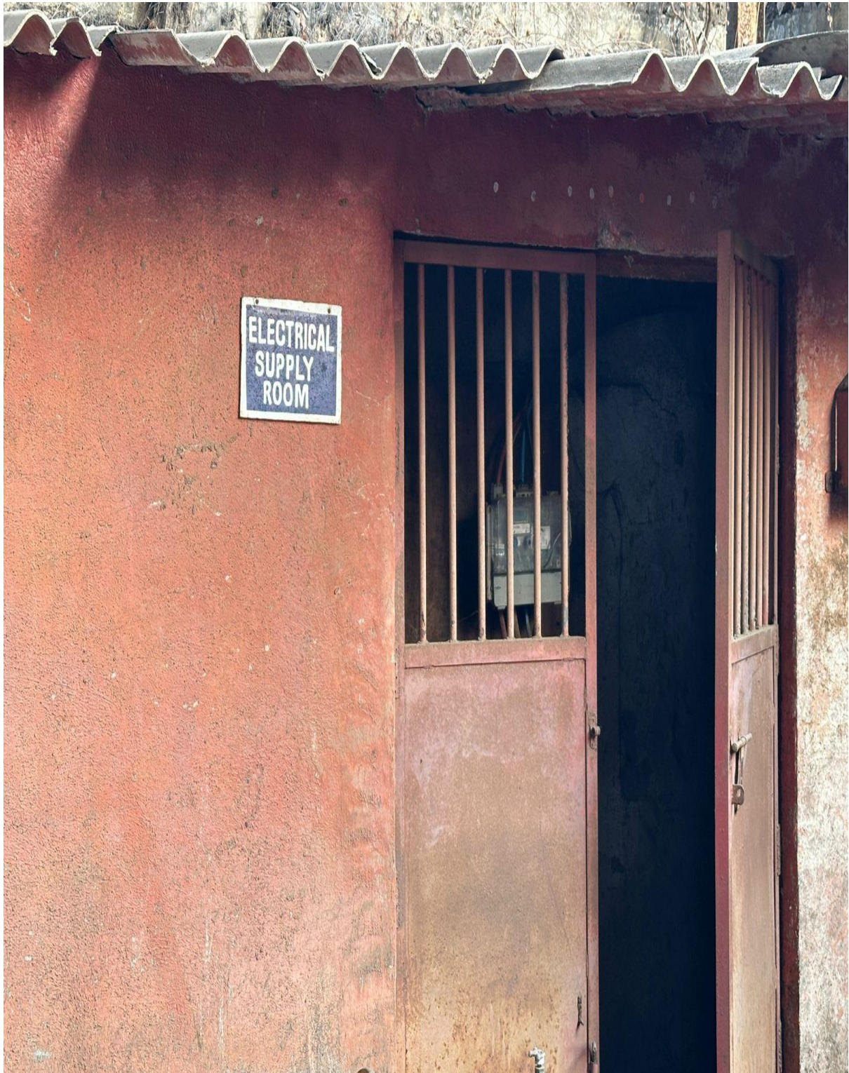
ELECTRICAL SUPPLY ROOM
