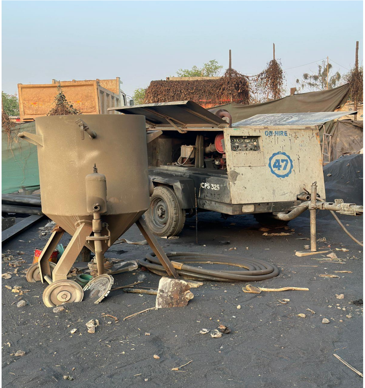
METALISING/BLASTING COMPRESSOR & HOPPER
