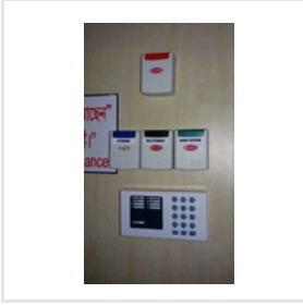
INTRUSION ALARM SYSTEM
