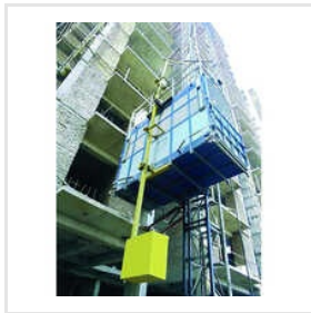
Passenger Cum Material Hoist Lifts
