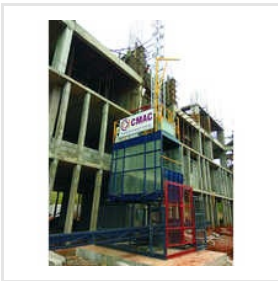
Industrial Passenger Cum Material Hoist
