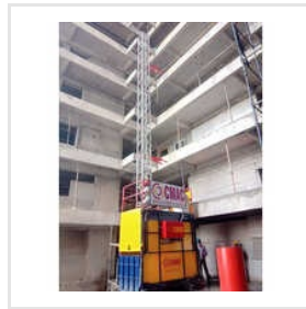
Construction Passenger Hoist
