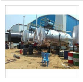
Bitumen Storage Tanks
