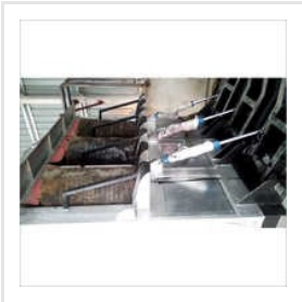
Bitumen Drum Decanter Plant
