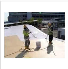
Roof Waterproofing Materials
