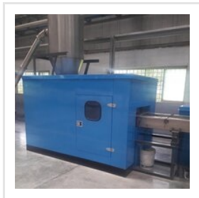
Pump Acoustic Enclosure
