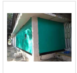
Compressor Acoustic Enclosure
