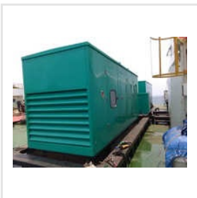
Generator Acoustic Enclosure
