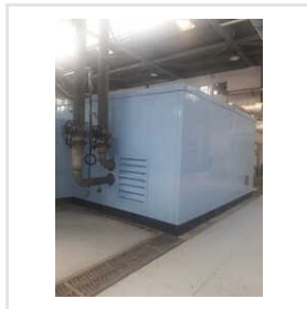
Chiller Acoustic Enclosure
