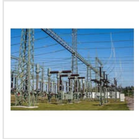
Electrical Open Axces Work Service
