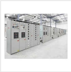
Electrical PCC MCC Distribution Panel
