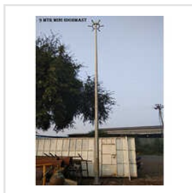
9 Mtr Octagonal High Mast Light
