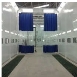
Bus And Truck Prep Station
