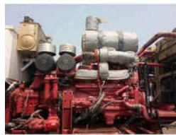
Manifold Energy Saving Insulation
