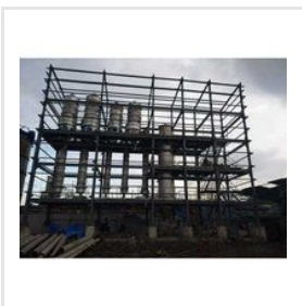
Evaporator Plant For Pesticide Industries
