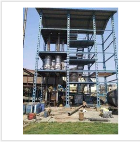
Salt Recovery Evaporation Plant
