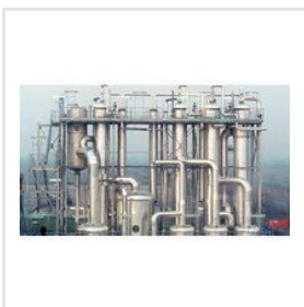
Multiple Effect Evaporation Plant
