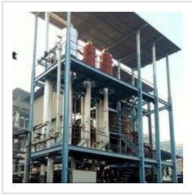
Multiple Effect Evaporation System
