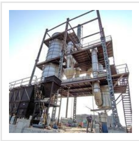
Spray Dryer Plant For Effluent
