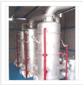
Zero Liquid Discharge Plant
