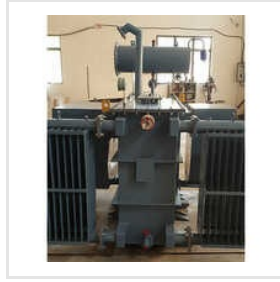
630 Kva 3 Star Transformer
