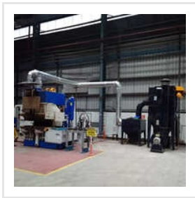
Fumes Extraction System For Gauging
