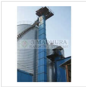
Grain Bucket Elevator Conveyor
