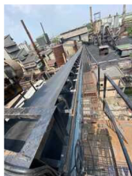
Belt Conveyor System
