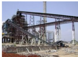
Coal Handling Plant
