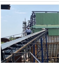
Coal Handling Plant
