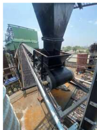
Belt Conveyor System
