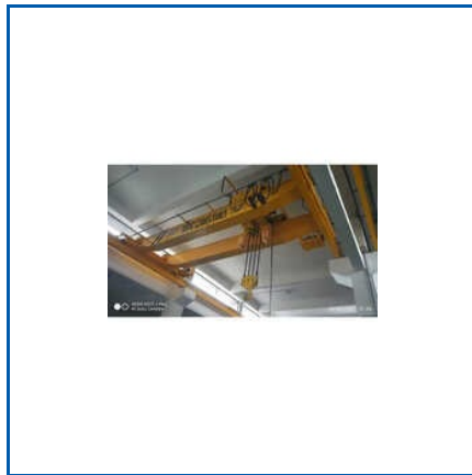
DOUBLE GIRDER EOT CRANES MANUFACTURE
