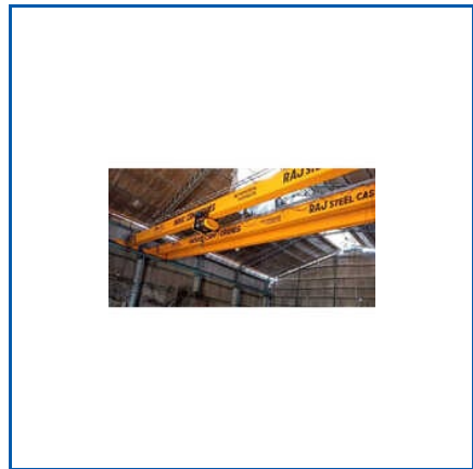
DOUBLE GIRDER EOT CRANE
