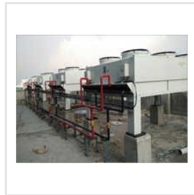
Air Cooled Condensing Units
