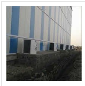
Cold Storage Chamber
