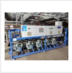
Compressor Rack System
