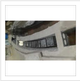
Underground Oil Water Separator
