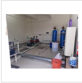
SBR Based Sewage Treatment Plant
