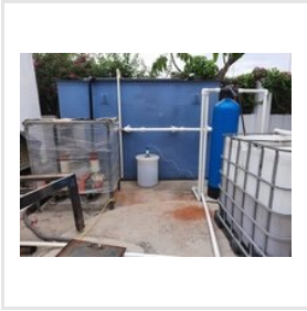
MBBR Based Packaged Sewage Treatment
