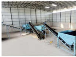
Industrial Coal Screener Plant
