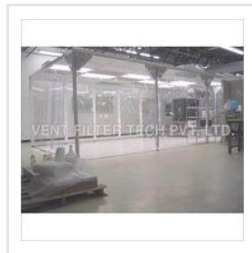
Soft Wall Clean Room
