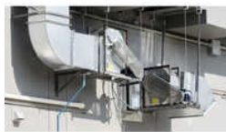
Basement And Kitchen Ventilation System
