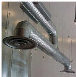
Industrial AC Duct
