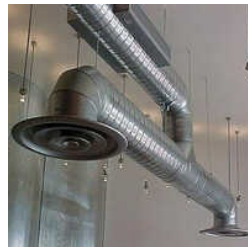
Industrial AC Duct
