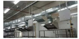
Basement Ventilation System
