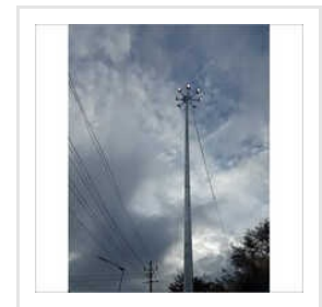
Electric High Mast Light
