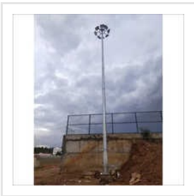
Street Light High Mast Pole
